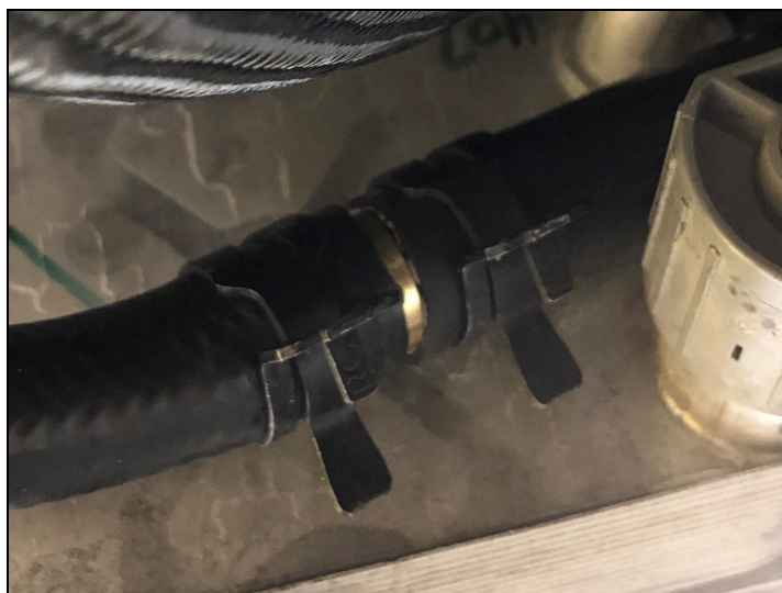
FIGURE 18 – Hose Coupler Installed with Clamps
